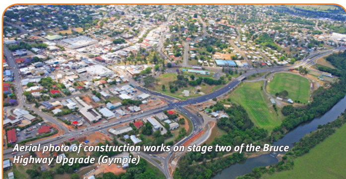
Stage two of the Bruce Highway Upgrade through Gympie looking north towards the Monkland Street intersection
